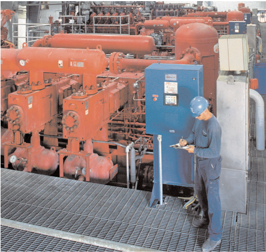
■ AGL Operator Danny Hebert stands beside one of the Jefferson Island's REMVue-500/A panels and checks off everything that is now right.
